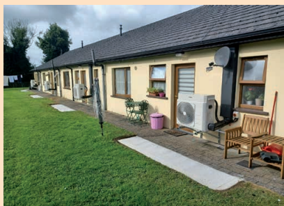
Recent air to water heating pumps installed at Clonmullion Retirement Village.
