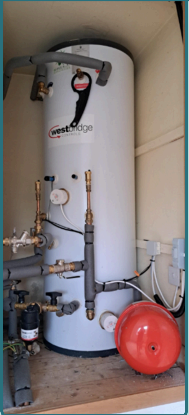
Hot Water Storage Tank
